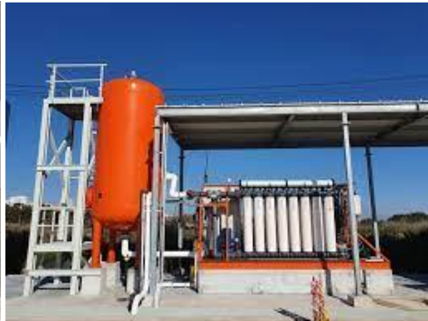
Filtration 10 - 20 m 3 /h
